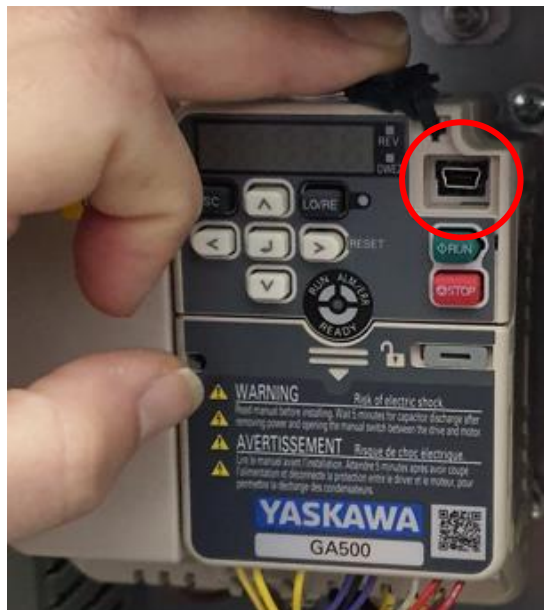
Figure 2: Cable Port Location
