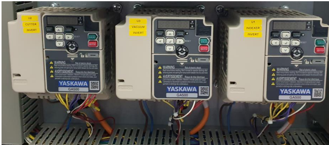
Figure 1: The Three Inverters
